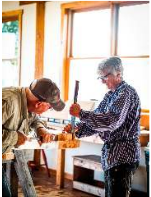
Above: Service learning volunteers spent a week at a time cutting the white pine timbers for the new Welcome Center, building community and connections along the way, Photo by Ben Finley.
